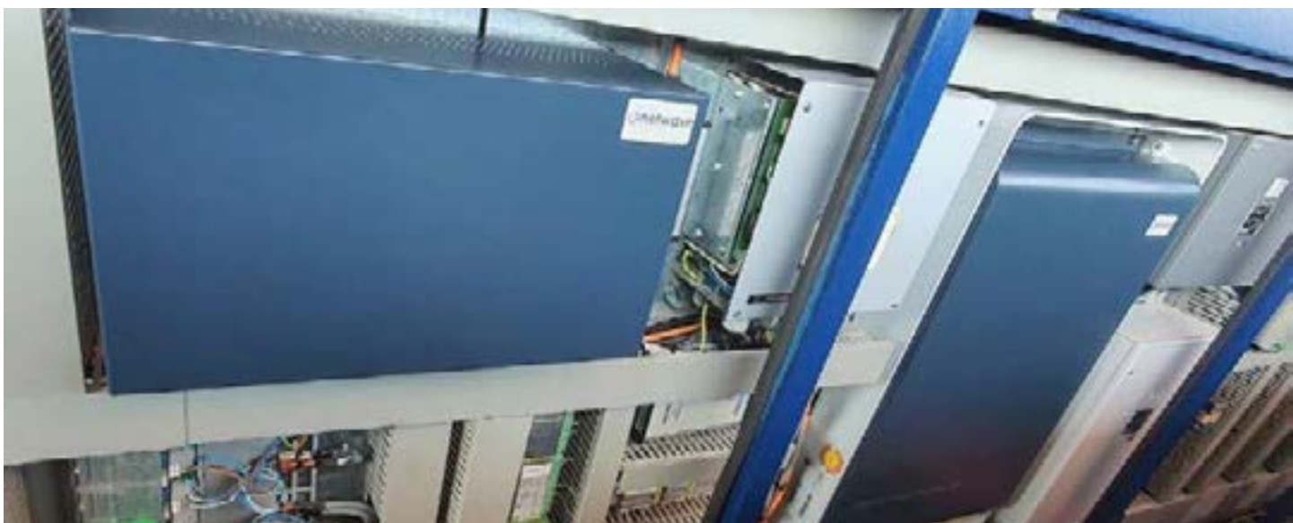
Installed NW6000 occupying previous VDR console
