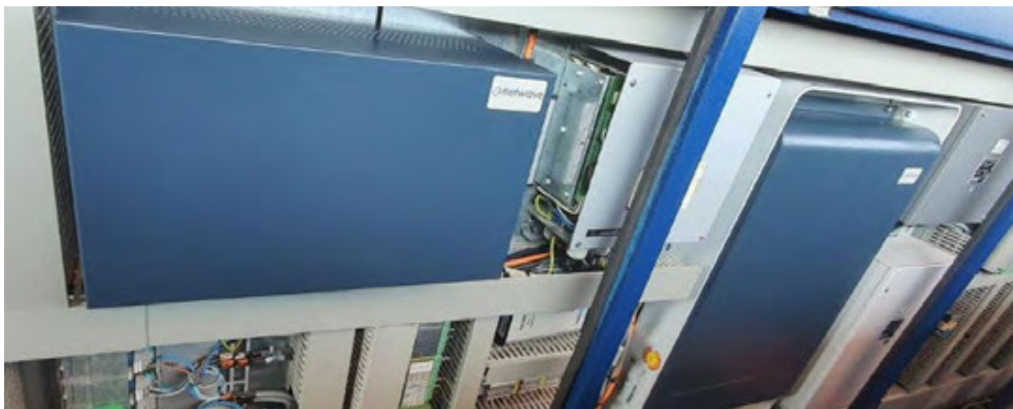
Installed NW6000 occupying previous VDR console
